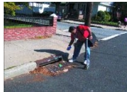
Field technicians were an unusual sight--even in New York City--as they traveled on Razor scooters with a mobile computer and treatment bag slung across their shoulders. After making a treatment, the technicians mark the catch basin.
